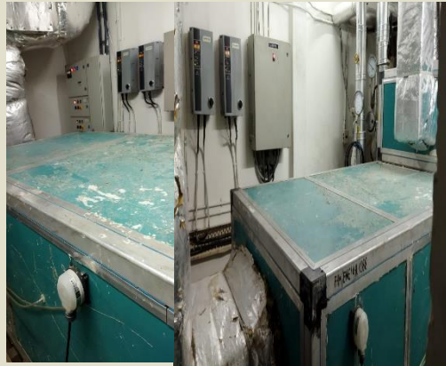
VFD Operated AHU's
