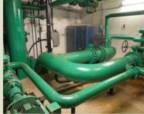
OTs chilled water supplies routed through main pump
