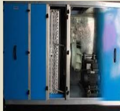
Ahu with EC fans
